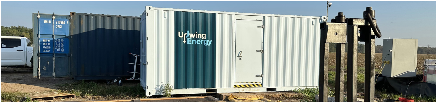
Upwing's temperature regulated Surface Control Container (SCC) housing electrical control equipment for the SCS at the wellsite
